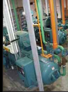
Shown left: (3) 350 horsepower ammonia screw compressors for a large freezing project
