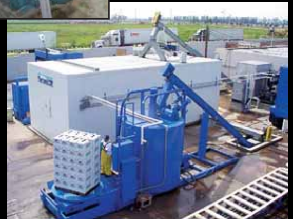
Shown below: system comprised of a 90 ton modular ice bin, plate icemaker and a Posi-jector™ for broccoli icing operation
